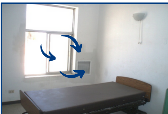
Figure 28. The patient room has mixed ventilation. Fresh air enters through an open window and is removed through a nearby mechanical exhaust ventilation system.
