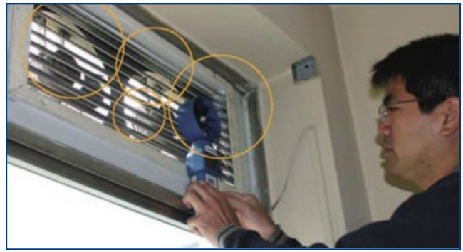
Figure 21. Anemometer to measure the velocity of air being exhausted from the room.
